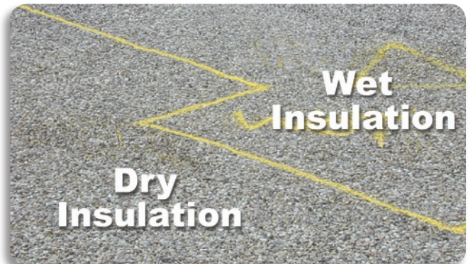
Control image, wet sections marked for removal
