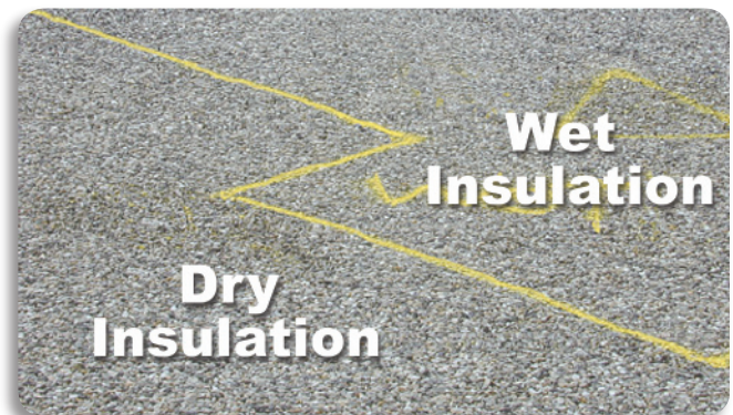
Control image, wet sections marked for removal
