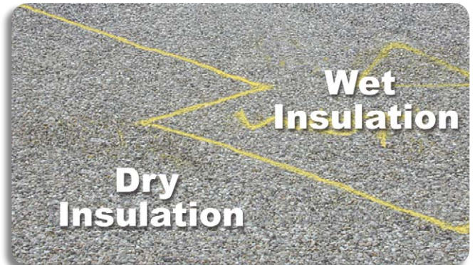
Control image, wet sections marked for removal
